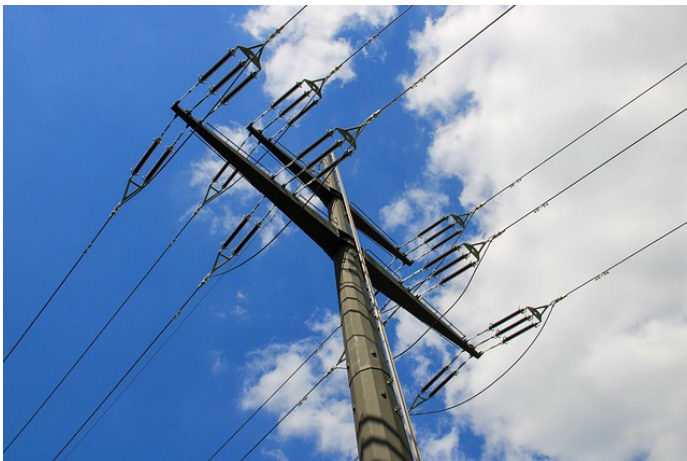
Electrical transmission lines (Source: NickyPe via Pixabay).
